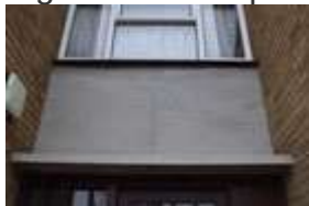
Fig 2 Asbestos panel on an external wall
