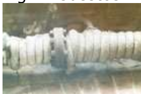
Fig 1 Asbestos insulation on a pipe
