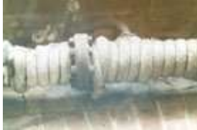
Fig 1 Asbestos insulation on a pipe
