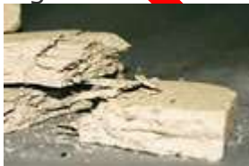
Fig 4 Pieces of Asbestos Insulating Board
