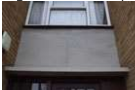
Fig 2 Asbestos panel on an external wall
